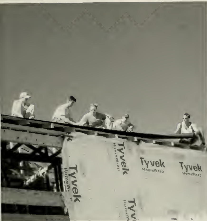
Left: Rodney Bower, a local construction contractor who travels with the organization, works with Erin Kahler, Rochelle Allison, Jason Moran, and Heather Zelle, to lay the roof sheeting.
