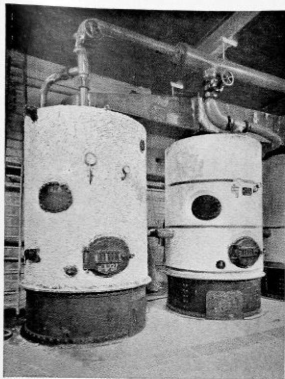
Fig. 8.—Battery of three coke-fired central heating boilers burning 16 pounds of coke per square foot of grate area; efficiency 85 percent
