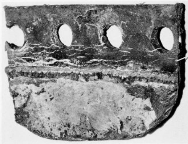
Fig. 4.—Example of welding employed to stop leakage through crack in boiler girth seam, discovered by visual method, which proved to be inaccurate in showing full extent of crack
