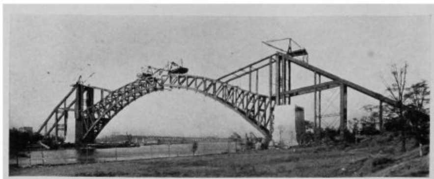
All but center panel of arch in place. Note part of approach viaduct in the background.
