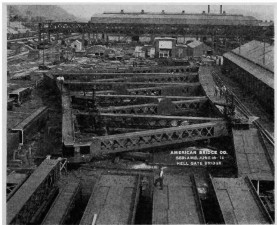
Section of Arch Truss temporarily assembled in Ambridge Yard to insure members connecting properly when erected in field.
