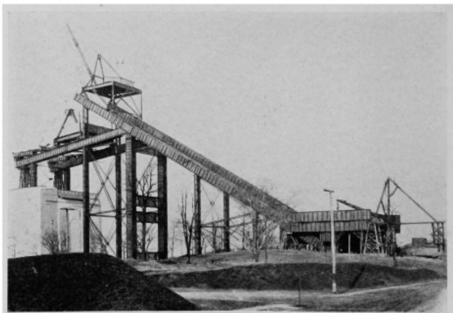
Back stay nearing completion composed of girders of the approach spans and stringers of arch spans. Note riling used for tower bracing. The back stay traveler is erecting the arch traveler.
