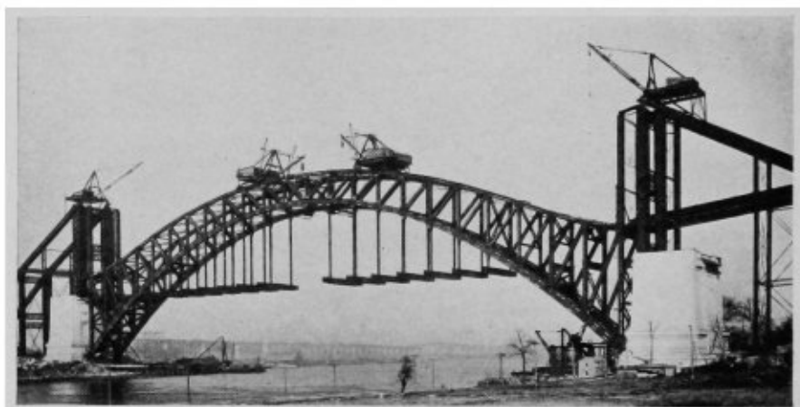
The arch closed and self-supporting. The upper back stay tie removed and the floor-beams mostly in place.
